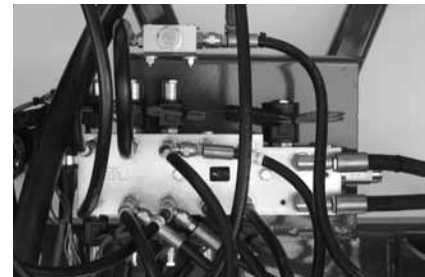
Hydraulic Control Directional Stack Closed Center Hydraulic System Set Up - Rear View
