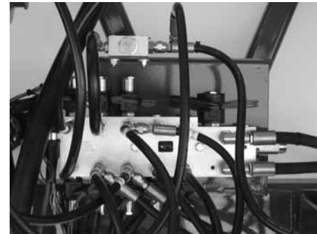
Hydraulic Control Directional Stack Closed Center Hydraulic System Set Up - Rear View
